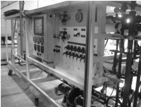
Figure 5. Equipment for secondary RO employed at the pilot testing at City of North Miami Beach Norwood WTP (Photograph by Sandeep Sethi 2009, with permission from City of North Miami Beach Utilities, FL)
