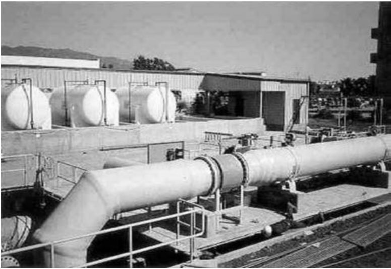
Figure 2. Pumping and Chemical Feed (Photograph by Bill Ferguson 2004, with permission from County of Santa Barbara Public Works, CA)
