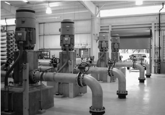
Figure 2. Ormond Beach WTP Vertical Turbine Membrane Feed Pumps
