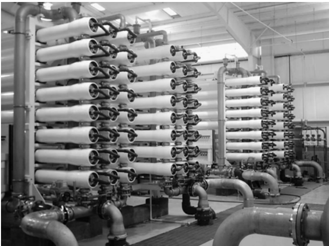
Figure 3. Ormond Beach WTP LPRO Membrane Skids
